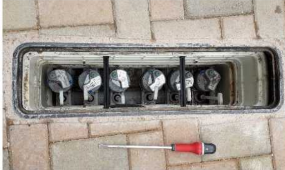
Image 3 - External (Manifold) Meter Installation
