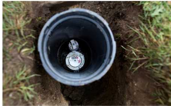
Image 4 - Externally Installed Meter
