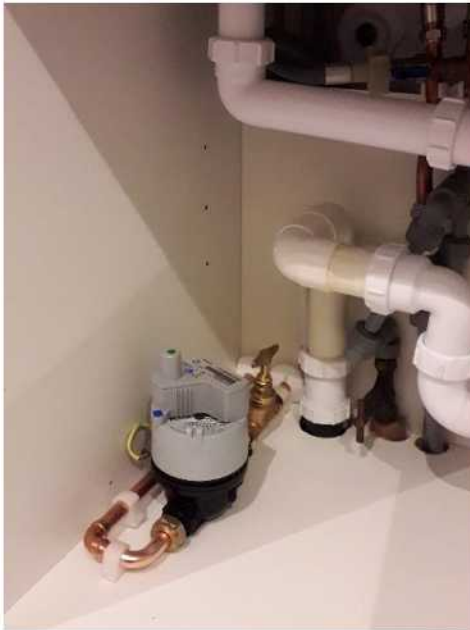
Image 5 - Internally Installed Meter
