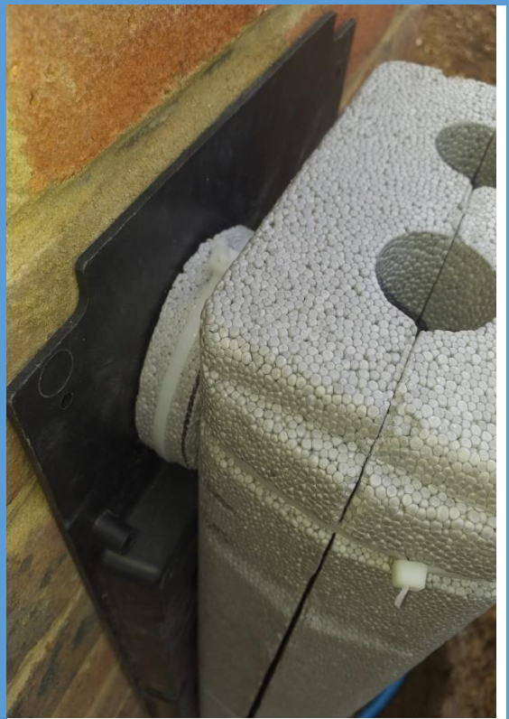
All pipework should be fully insulated.
